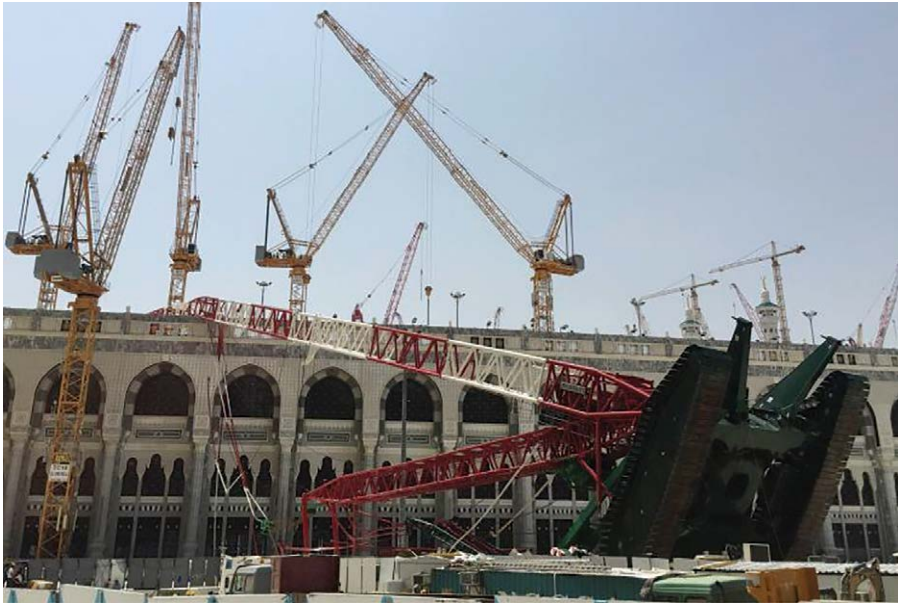
Fig. 11.4. Crane collapse during Hajj, September 2015, Ka'ba. Source: Mustafa Acar
